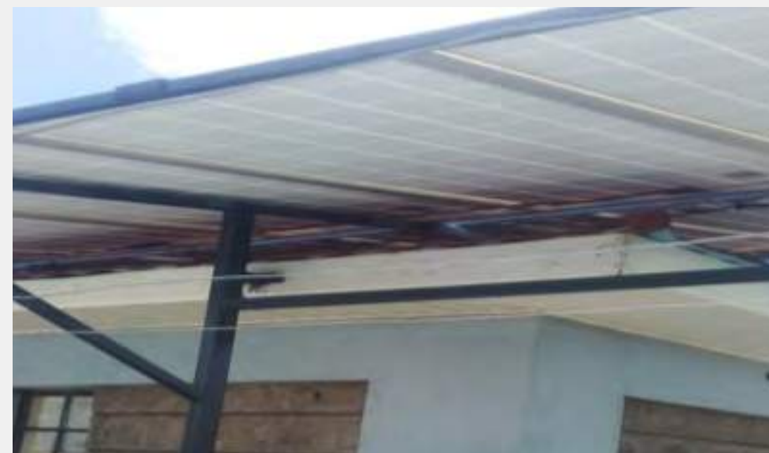
Solar panels installed
